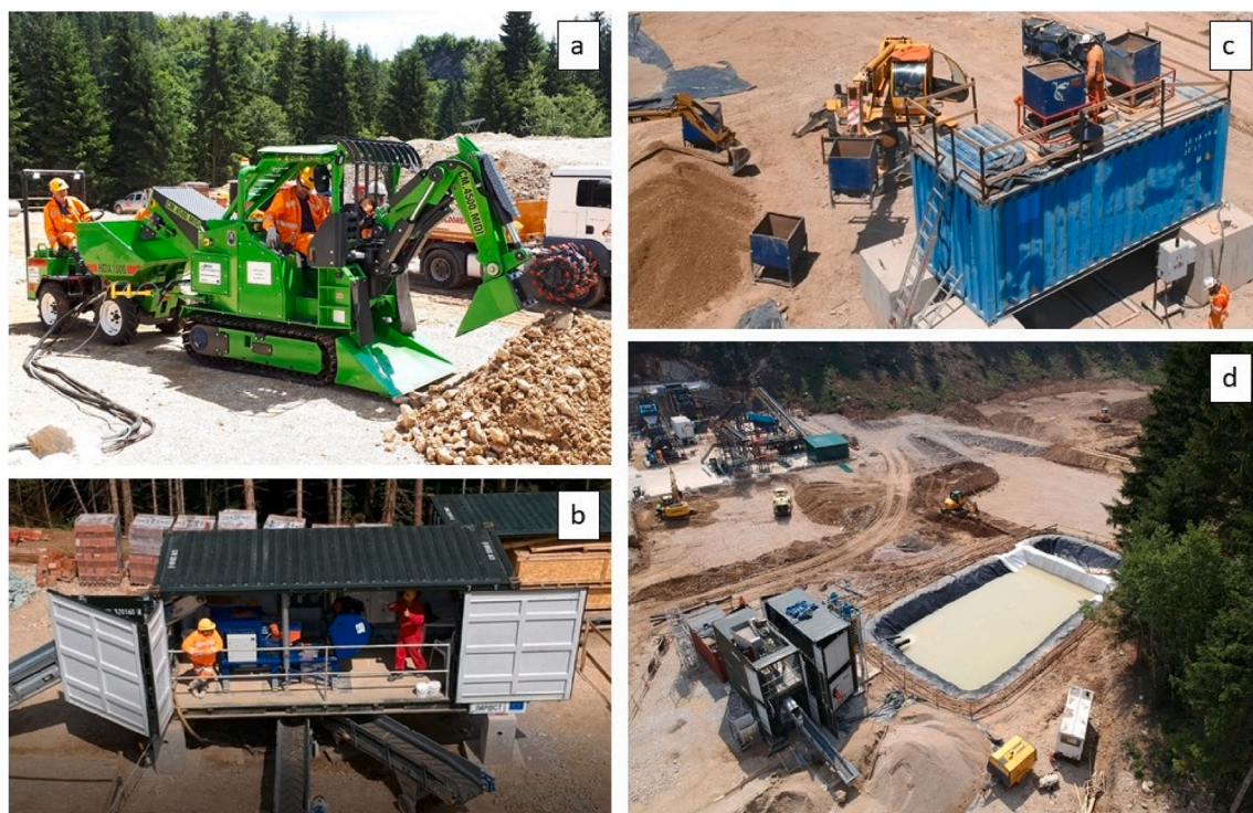
Fig. 1. The containerised technical solutions deployed at the first test site (Olovo) in Bosnia and Herzegovina. Equipment comprises (a) a prototype machine for selective underground mining, (b) XRF ore-sorter unit, (c) comminution unit, and (d) gravity separation plant (throughput 5 ton per hour) in the foreground – the full scale processing plant is under construction in the background. Published with the agreement of Metal Innovations, Extractive Industry, Rados International, University of Exeter and Mineco.
